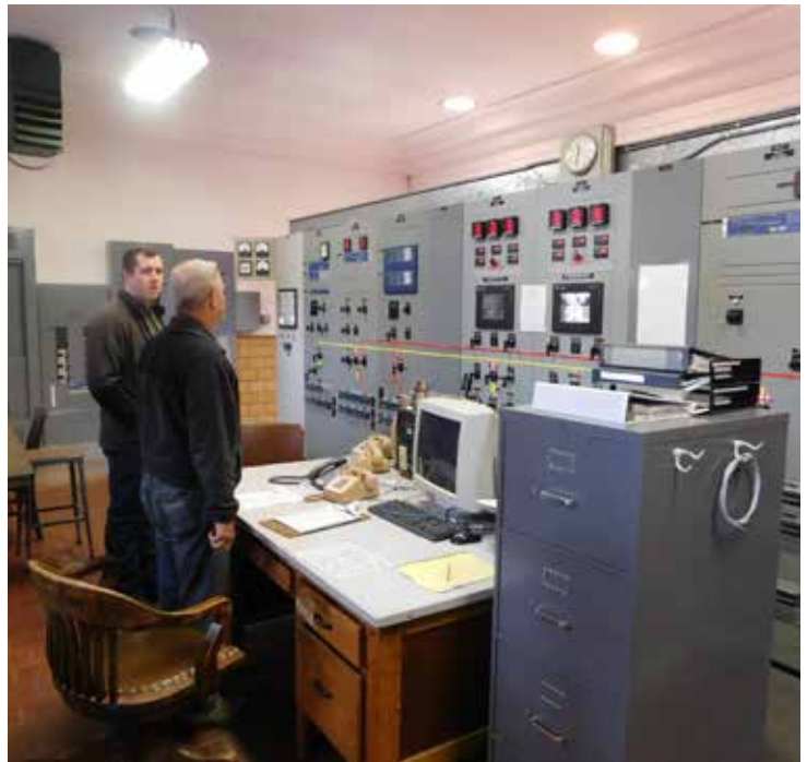
Ben Beckman and Jeff Buettner look over the control panel for a hydro-power station at Johnson Lake.
